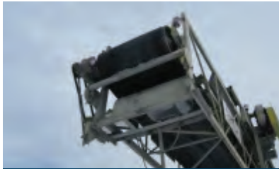
Automatic Lubrication System on Head Pulley of Belt Conveyor
