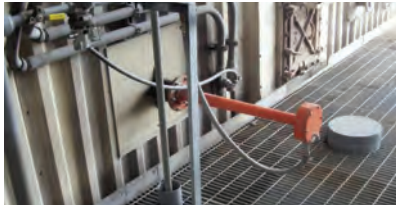
Sonic Horn Mounted to Vessel to Promote Material Flow
